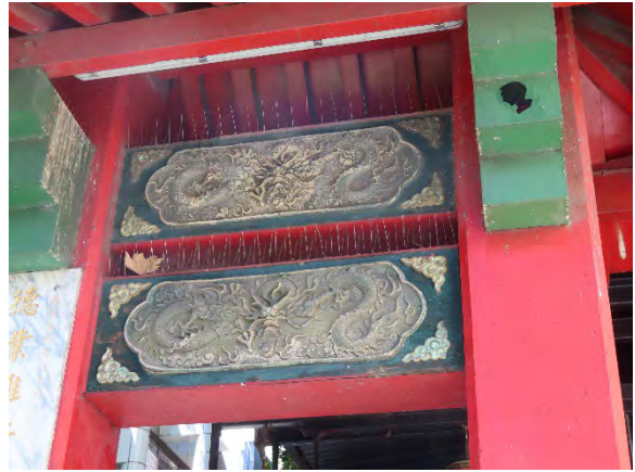
Figure 4.9 Decorative moulded panels E and E featuring motifs in fibreglass at the western bay.
