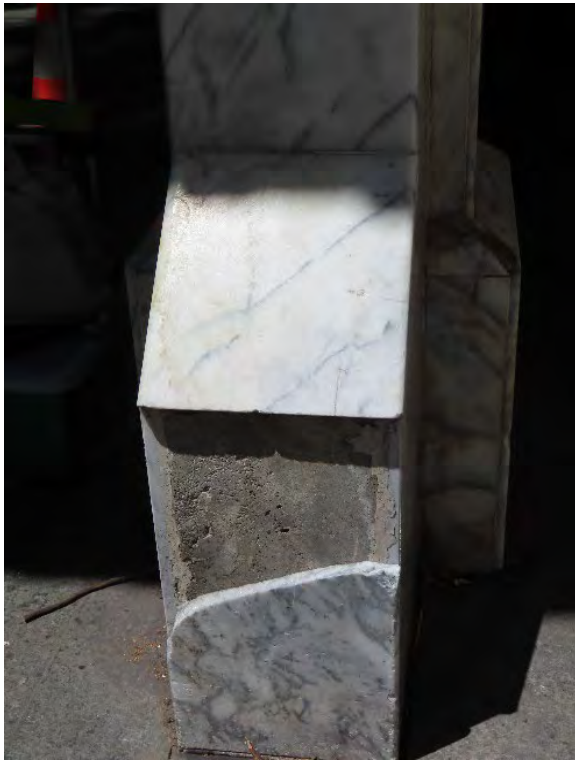
Figure 4.26 Broken marble plinth.
