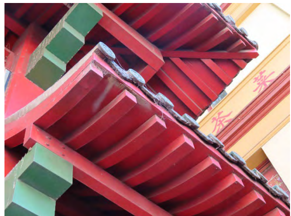
Figure 4.44 View of the underside of the upper and lower roofs showing delaminating plywood soffit.
