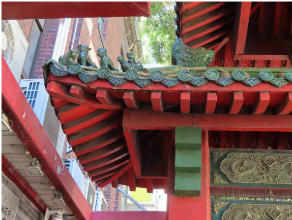
Figure 4.14 Symbolic ceramic capping tile figures on the hip of the lower roof—eastern bay.
